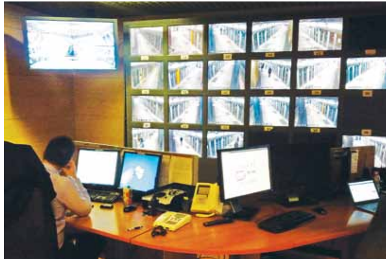
The pilot installation of networked CCTV with intelligent analysis went live in the Torino metro control centre in March.
